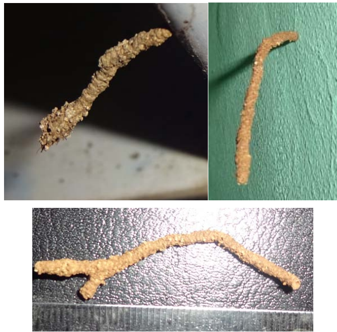
Fig. 10: Suspended mudtube over the concrete wall
