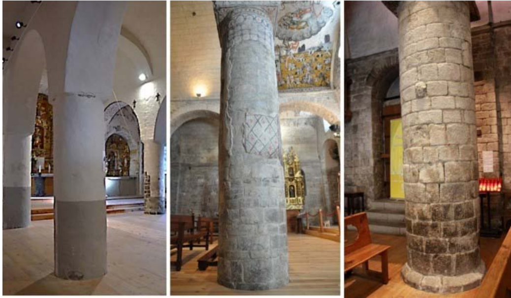
Fig. 1: Deformation of the pillars: Santa Eularia d'Unha, Santa Maria d'Arties and Era Purificacio de Bossost
