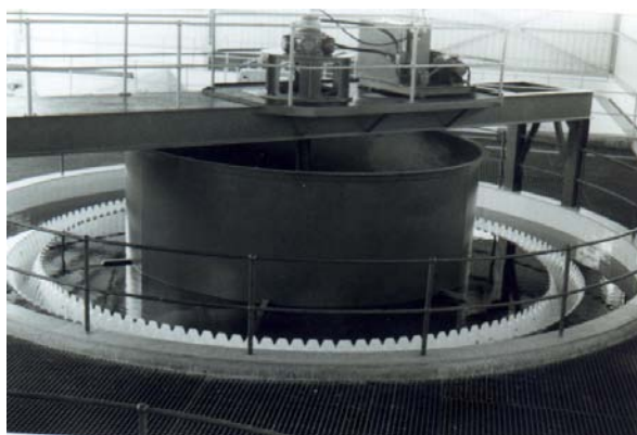
Figure 23: The Saulspoot waterworks – the HR clarifier, design capacity 10 ML.d -1
