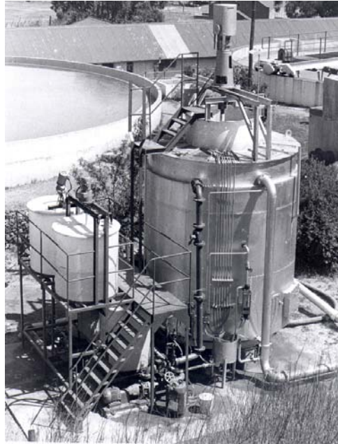
Figure 21: Installation of the second pilot HR clarifier at the municipal waterworks of the City of Bethlehem
