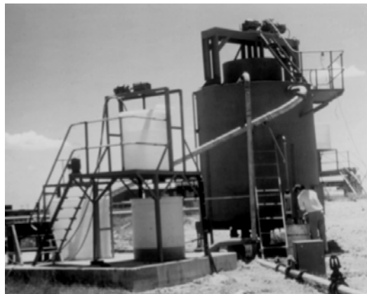
Figure 20: Installation of the pilot HR clarifier at the RWB Zuikerbosch waterworks
